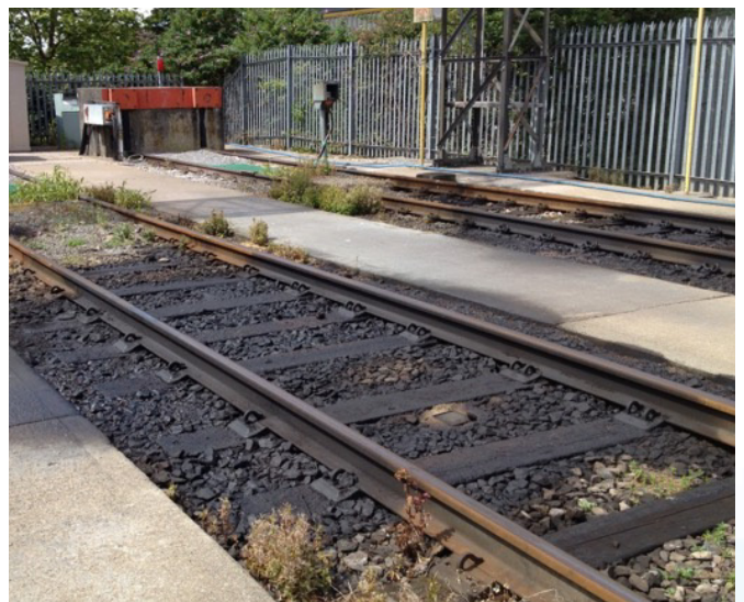
A oil spill impacting a railroad ballast. PetroFix can be used quickly and effectively to mitigate against the effect of small-scale spills such as these.
