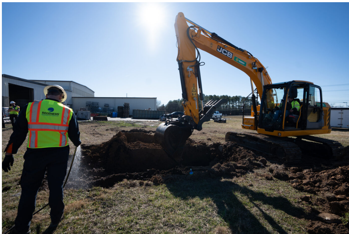
Regenesis' remediation solutions are used at manufacturing sites, airports, military bases and other locations with heavy soil pollution
