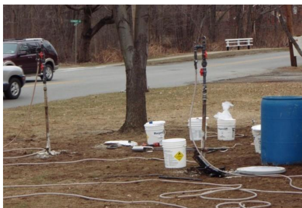
Figure 4. Permanent Injection Points
