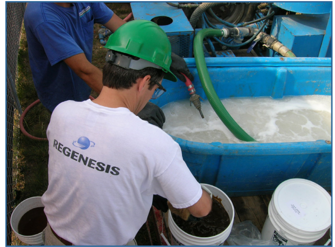
3-D Microemulsion was applied on-site to treat high levels of carbon tetrachloride.
