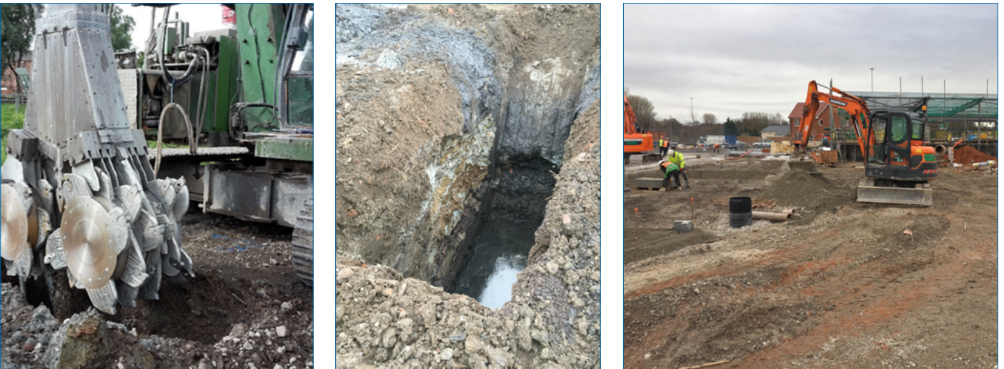
Fig. 9,10 and 11 - Installation of the soil-cement stabilisation panels by Deep Soil Mixing Ltd
