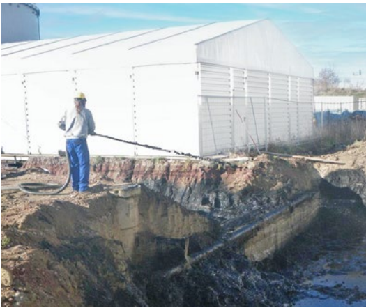
A field services applicator spray-applies PetroFix to the walls and base of the excavation.
