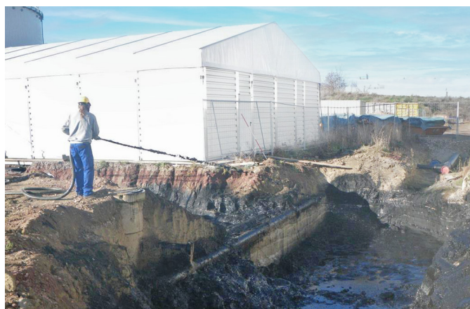
A field services applicator spray-applies PetroFix to the walls and base of the excavation.
