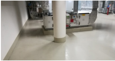
The injection work was completed in a subterranean car park with precautions taken to ensure a clean working environment and no damage to the existing machinery.
