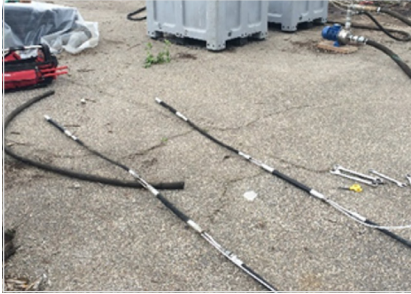
Above: Inflatable packers were used for isolating discrete vertical injection zones during the application of PetroFix.
