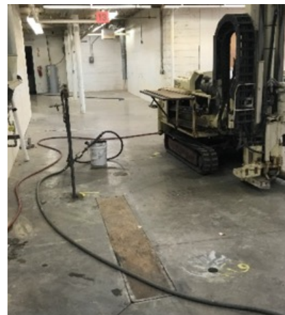
PlumeStop Injected at Multiple Points Simultaneously
