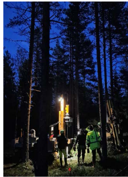
Figure 4 The barrier installation was carried out over nine weeks, despite the decreasing daylight hours and challenging weather conditions in the final weeks of the works.
