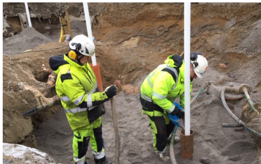
Fig. 1 (top) Targeted excavation around UST Fig. 2 (right) Installation of injection wells by RGS Nordic
